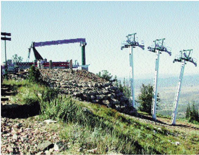
This detachable quad from Doppelmayr/CTEC was installed at Beaver Creek. The new lift will cut the ride time up to Larkspur Bowl from 11 minutes to 5 1/2.
