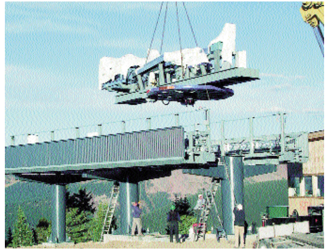
For its new Super Gauge Express, Winter Park has purchased enough clean, renewable wind energy to run this Leitner-Poma detachable quad for the season.
